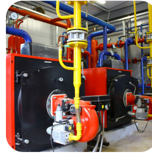
Central Heating and Cooling Systems
