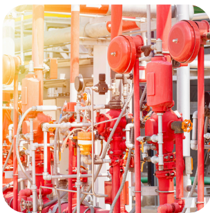
Fire Protection Systems
